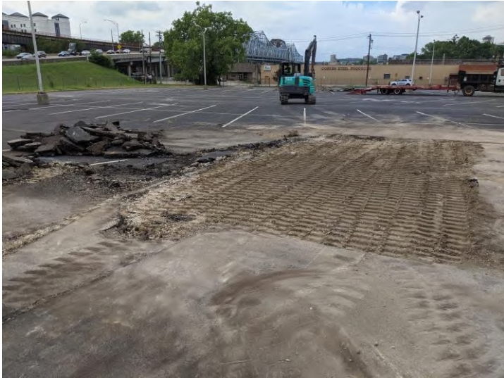
Photograph 5: View of the backfilled cavity in Survey Area #6 at completion of excavation.
