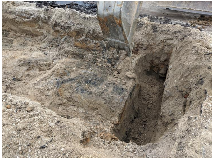
Photograph 4: View of the steel tank ("Tank #2") uncovered in Survey Area #6 (Bonded Station west).
