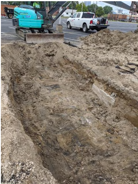
Photograph 3: View of the steel tank ("Tank #2") uncovered in Survey Area #6 (Bonded Station west).
