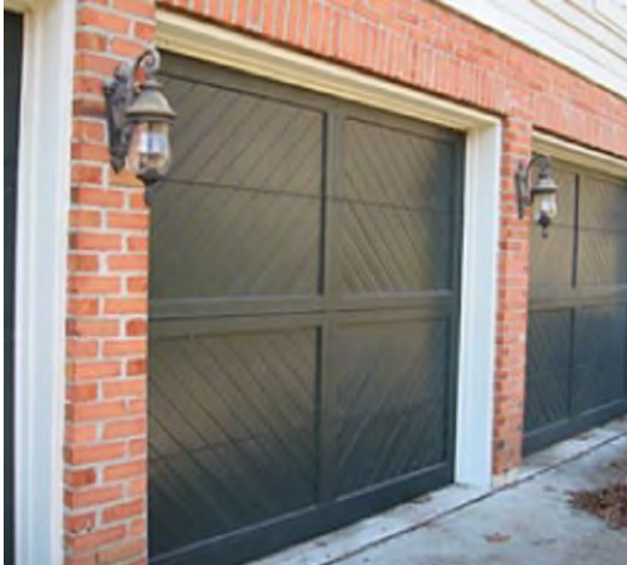
Appropriate replacement sectional roll-up garage doors
