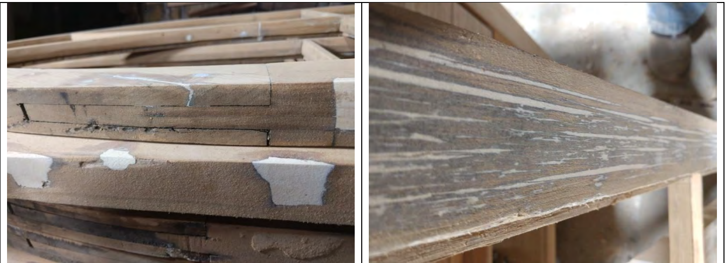
Photos of same window showing in-progress repair with epoxies and wood fillers.
