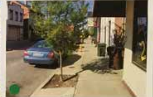
4 PEDESTRIAN ACCESSIBILITY Broken pavement, inadequate ADA ramps and trash cans often restrict the clear zone for pedestrians
